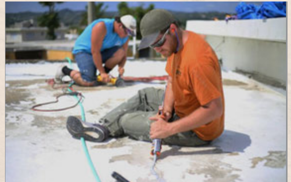
First Year Members Eli Schmit and Frankie DiVito provide concrete roof repair on a home affected by Hurricane Maria in Puerto Rico.
